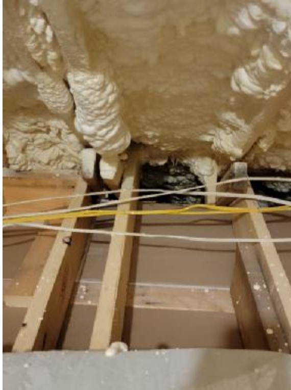
Attic insulation on sheathing none on ceiling
