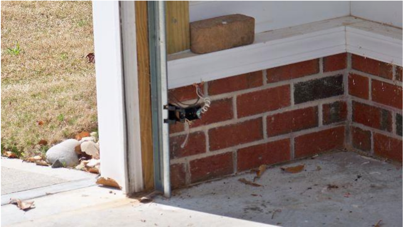
Garage & Carport infrared too high
