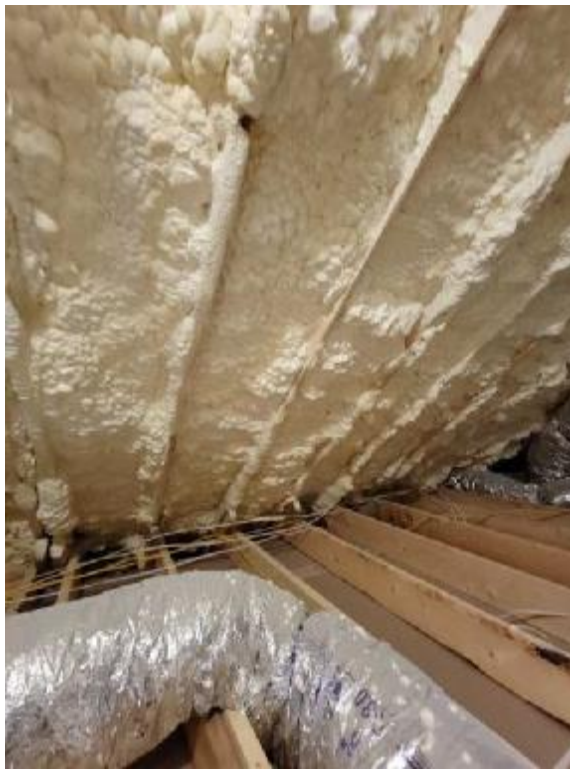
Attic spray foam insulation
