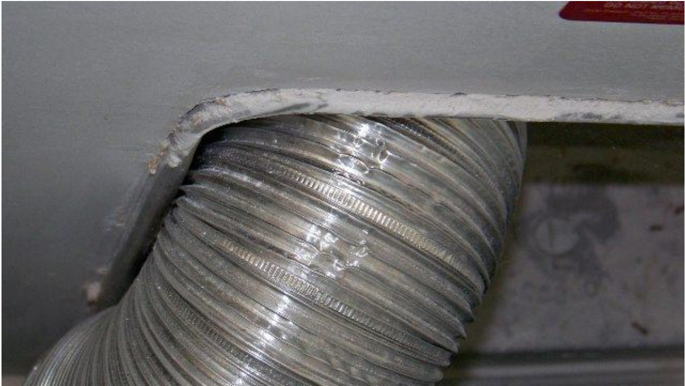
Kitchen & Laundry flex dryer duct
