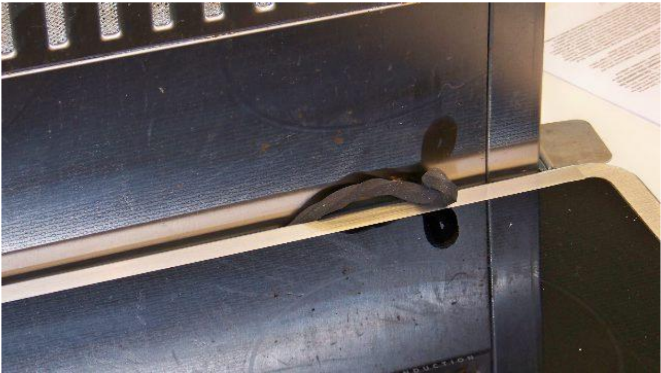
Kitchen & Laundry loose gasket on range top vent
